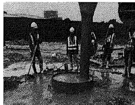
In situ construction of bored pile in Kajang for Package V8 of the Klang Valley Mass Rapid Transit Sungai Buloh-Kajang Line project undertaken by our Group
