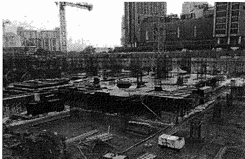
Basement works using the bottom-up method for Parcel C of the KL Eco City Project at Jalan Bangsar, Kuala Lumpur as undertaken by our Group
