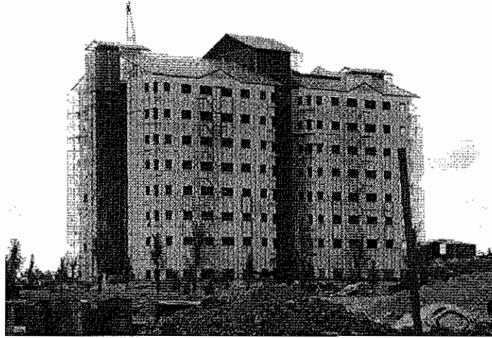
Construction of a police training centre in Terengganu undertaken by our Group
